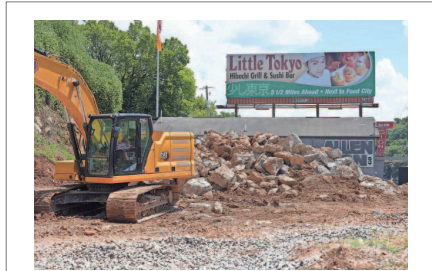
What was once the site of Burger Boys along Chapman Highway is now being turned into a new entrance for Kern's Food Hall.
